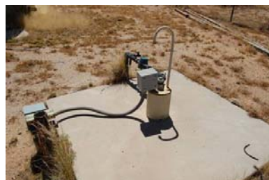
1000 Gallon Pressure Tank with Pressure Switch
